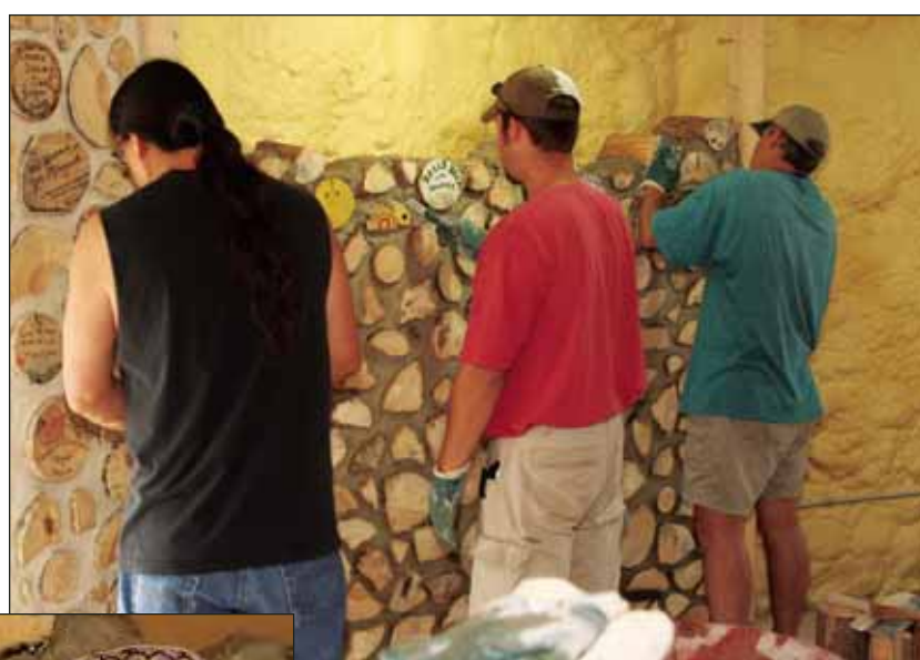
Photos courtesy of Sylvia Cornelius-Waupoose Top: Rod Hill, John Habeck and Micheal Finney work on setting up a wall made of cordwood. Left: Sylvia Cornelius-Waupoose decorated this cordwood log for the sugar shack under construction.
