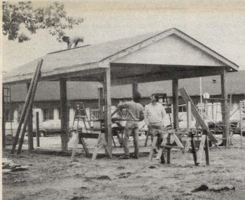
Randy Jourdan and Larry Cornelius look on as Aloyious Jourdan works on the roof of a shelter for the elderly located across the entrance of the Anna John Nursing Home next to the Oneida Health Center. This project is a joint venture between the WCC crew and the Public Works/Building and Grounds Department. The shelter has now been completed.
