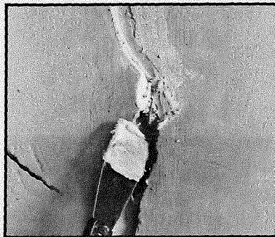
Mix a batch of plaster and fill the cavity. Allow a drying period of 24 hours. Shrinkage may occur during drying.
